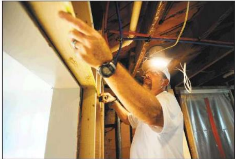
Technician Doug Beardsley of Mr. Handyman and H.M. Remodeling of Greater Fairfield County, works on installing a new kitchen in a home in Fairfield on Wednesday.
